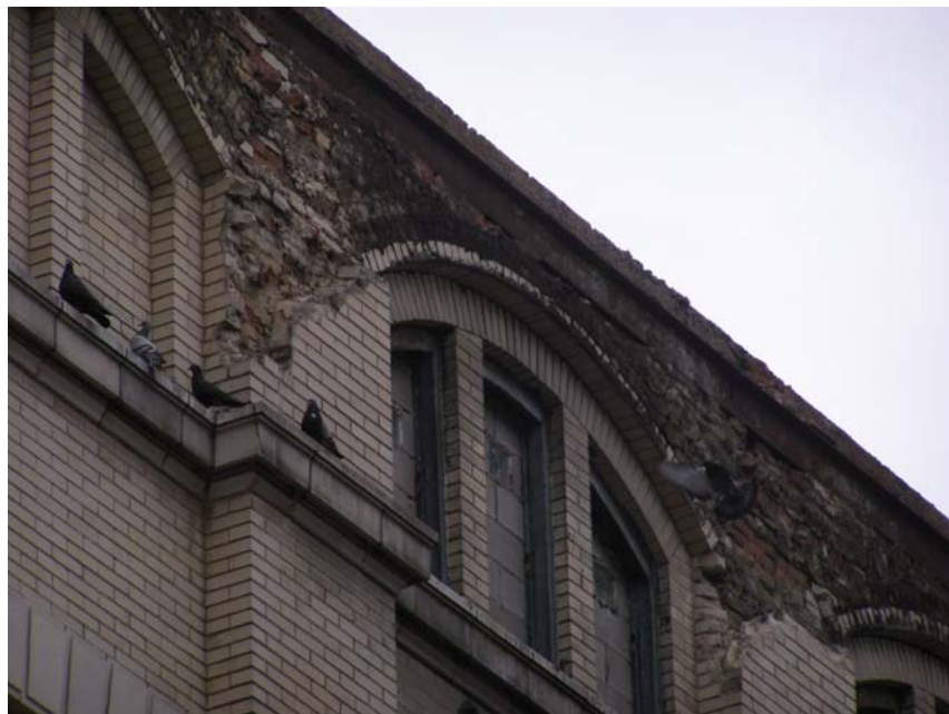
Photo 3 shows failed brick on façade.
